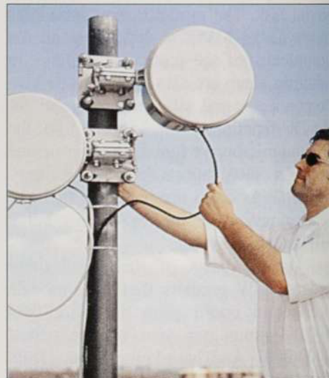
Photograph of a 38 GHz antenna used by WinStar in point-to-multipoint wireless links.
