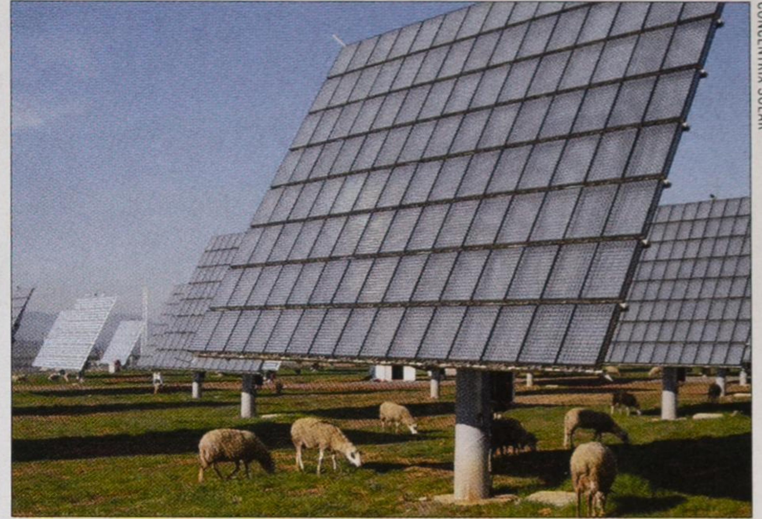
Solar farm: the design of most concentrated photovoltaics trackers allows mixed use of land, as this image from Concentrix Solar's power plant in Puertollano, Spain, clearly demonstrates.
