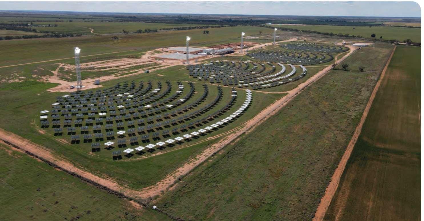
► Figure 3. Construction of the 4 MW electricity plus 3 MW/ 50 MWh storage project near Mildura, Australia, is nearing completion. Each solar field utilises nearly 300 mirrors to concentrate light onto a central receiver. (The cold and hot water pits can be seen behind the fields of mirrors.)
