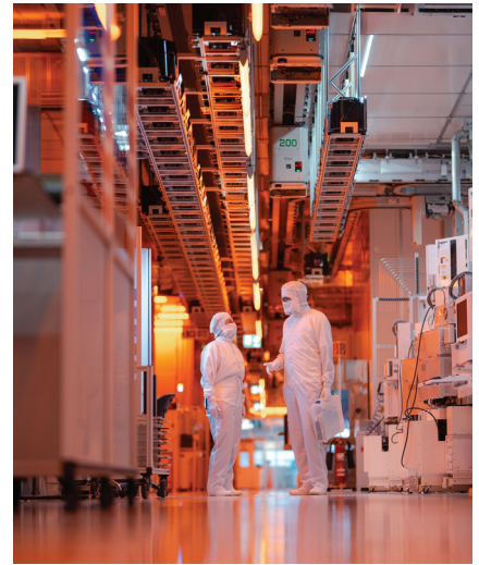
➤ Dresden cleanroom, 300 mm cleanroom at Infineon Dresden’s existing site. [Infineon]
