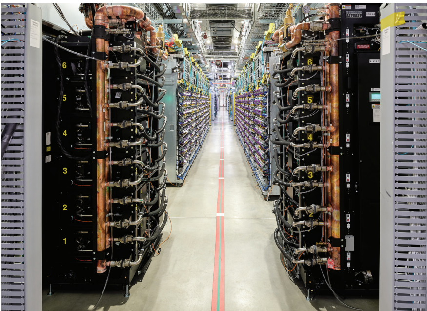
➤ Keeping cool: a Google data centre aisle, with coolant distribution units, at New Albany, Ohio. [Google]
