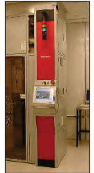
Microsemi has a Centrotherm HV 100 high temperature implant anneal system in its power chip fab in Bend, Oregon. This tool is capable of operating at up to 1700°C
