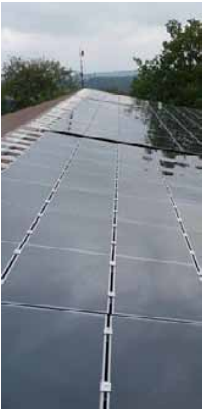
Rooftop array using Q.SMART modules on industrial building in North Rhine Westphalia, Germany
