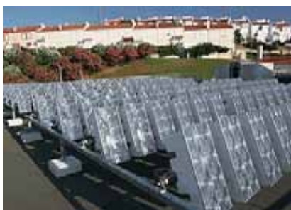
Emcore Soliant 1000 rooftop system
