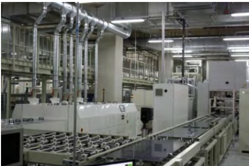
TSMC Solar facility in Taiwan
