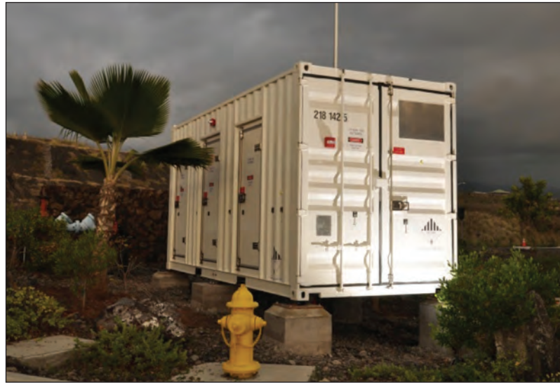
A typical installation of a containerised energy storage system
