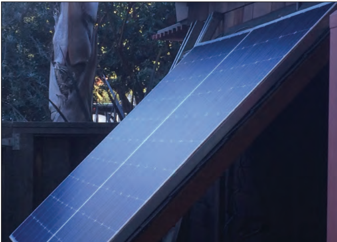
Figure 4: 2, 260Wp Giga Solar modules installed on a test roof
