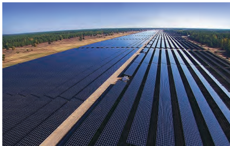
Thin-layer in rows: solar project developer Belectric has built Europe’s biggest photovoltaics power plant in Eastern Europe using cadmium-telluride modules by First Solar.
