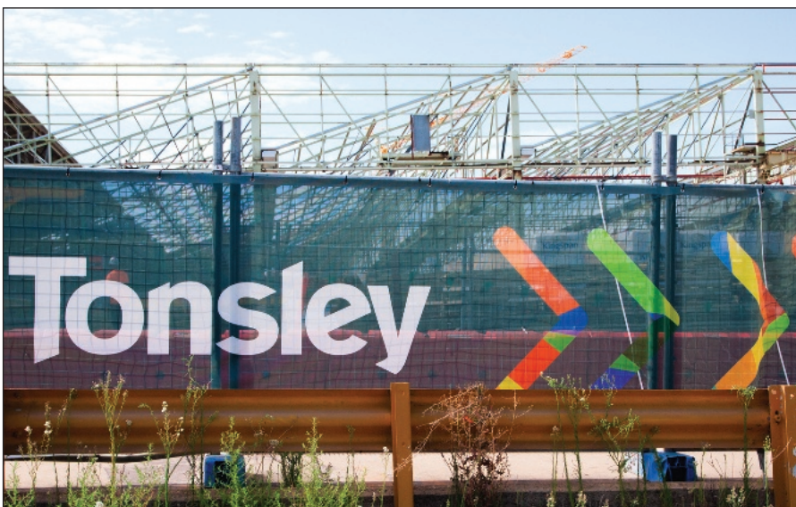
Tonsley during early construction. The sawtooth roof will soon be covered in a massive solar panel array.
