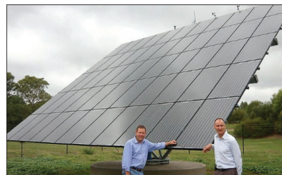
One of the 80 kWh tracking arrays lining the road to the Jacob's Creek visitor's centre.
